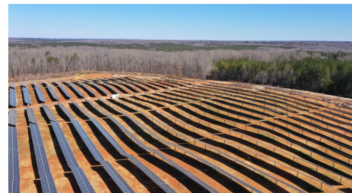
EPC Contractor Virginia – 17 MW
